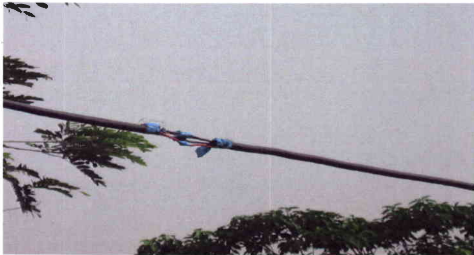
Photograph showing technique used to steal power
