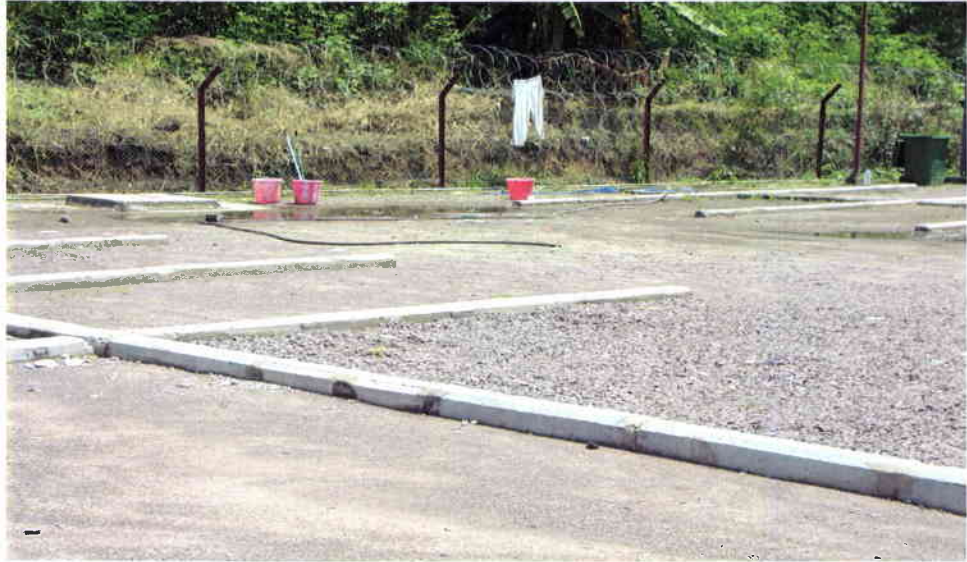
Photograph 1: Example of poor quality work
